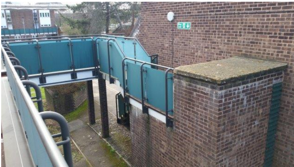
▲ F.10 Bare concrete roof to bin shoot allowing rainwater penetration
