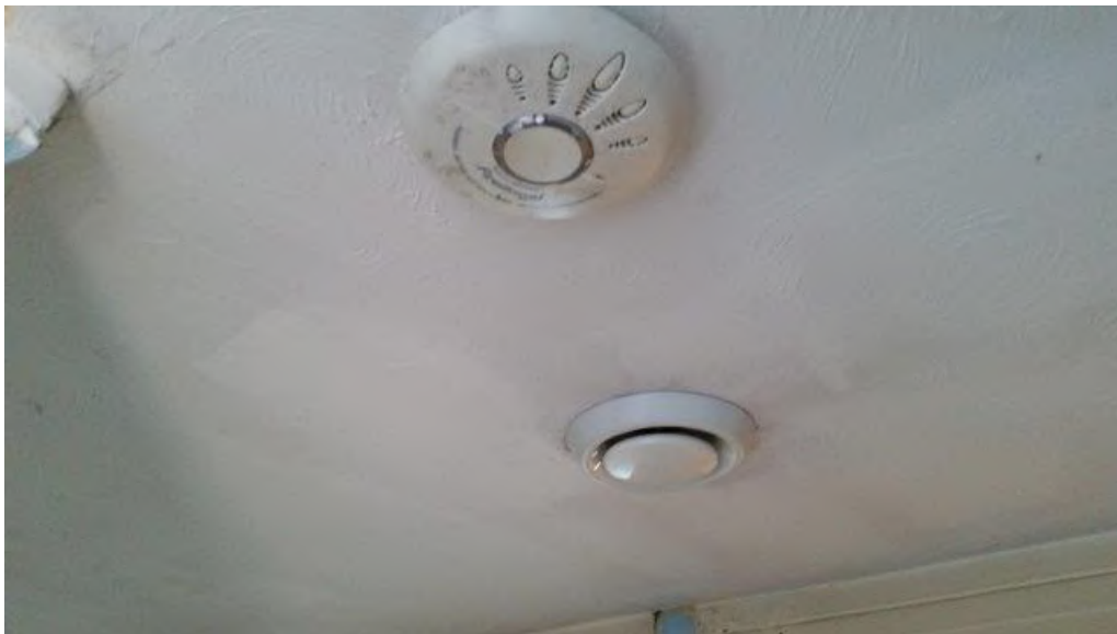
▲ F.32 Redundant fittings left
