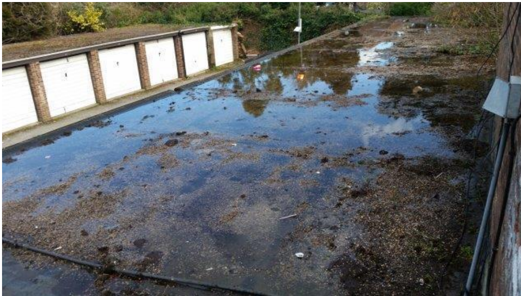
▲ F.30 Garage block roofs saturated, not draining and allowing vegetation to grow
