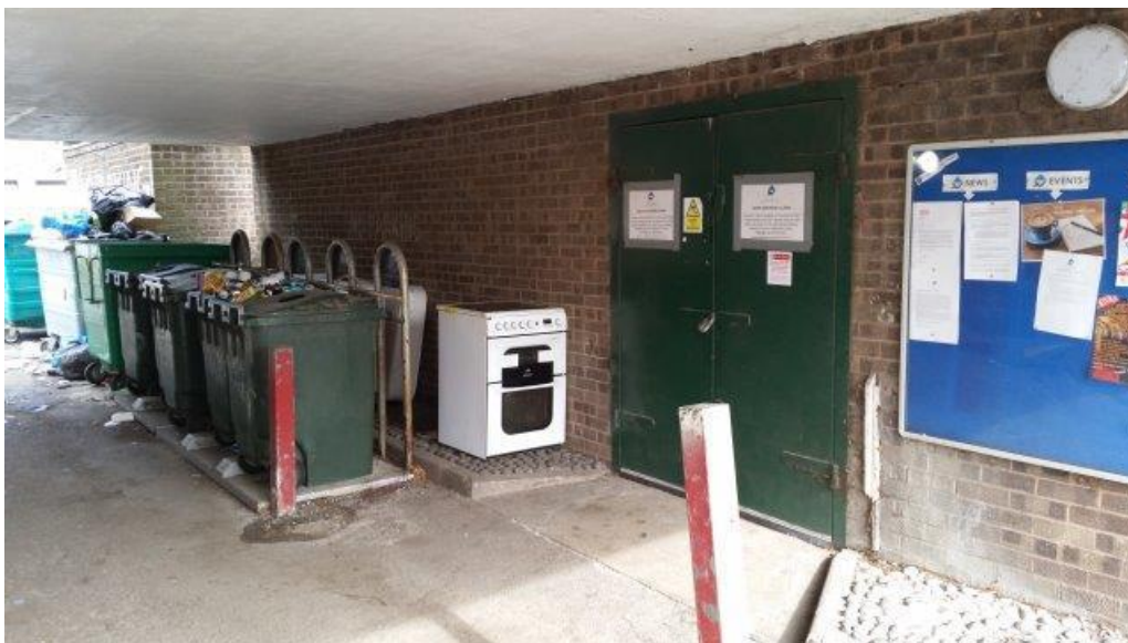
▲ F.44 Fire risk from furniture dumped under overhang soffit
