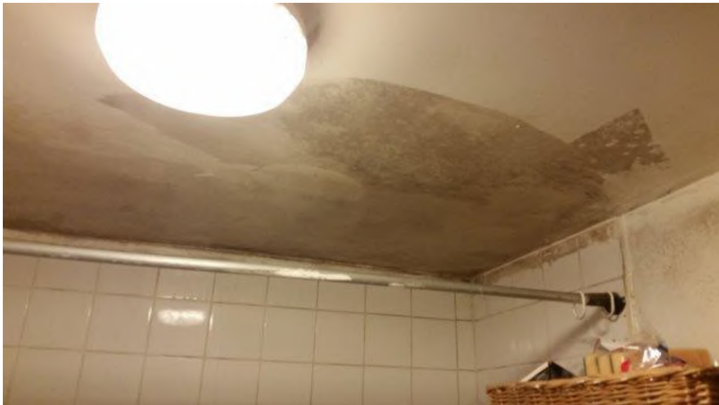
▲ F.37 Severe condensation to many bathrooms
