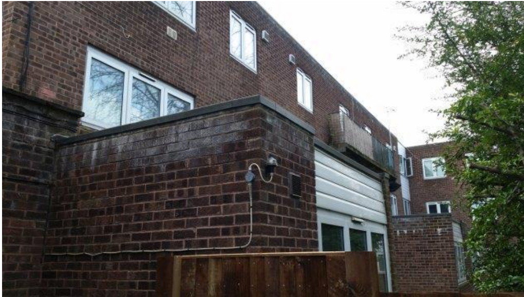
▲ F.13 Parapets in poor condition
