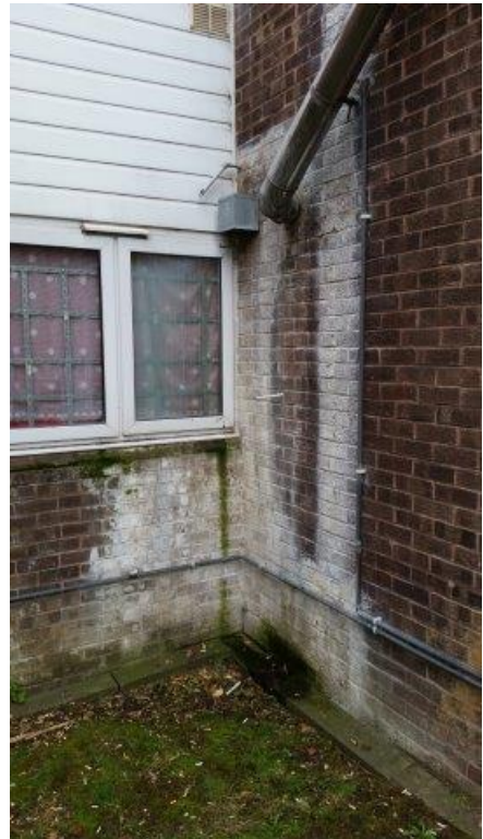
▲ F.18 Severe staining to Block 1
