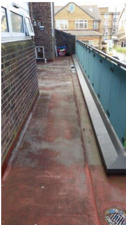
▲ F.23 Walkway covering discolouring and losing tactile texture
