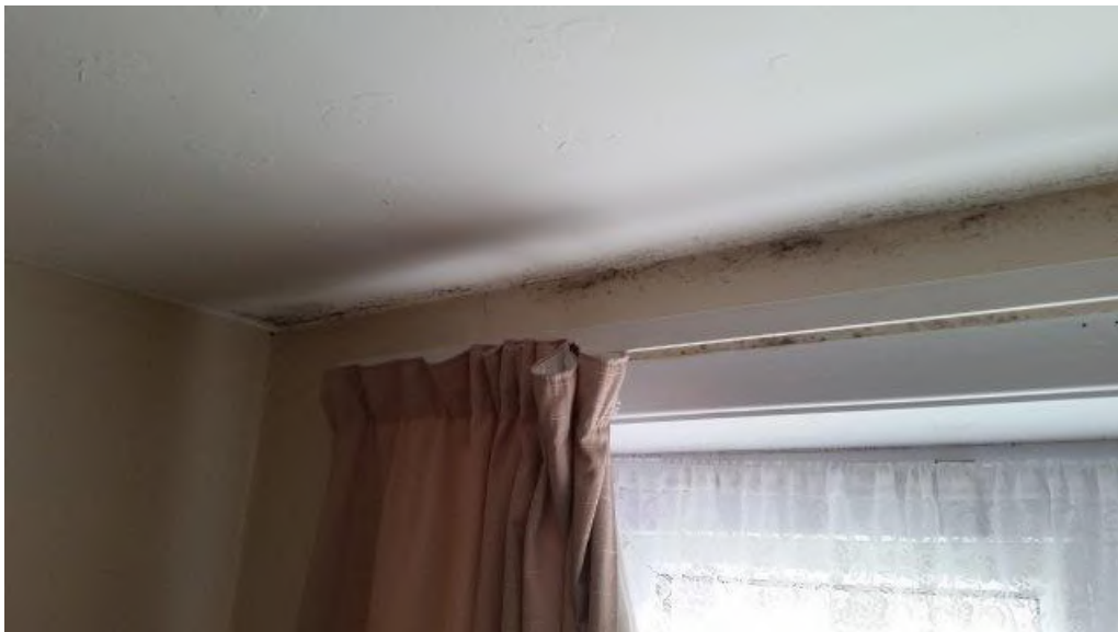
▲ F.34 Condensation prevalent throughout
