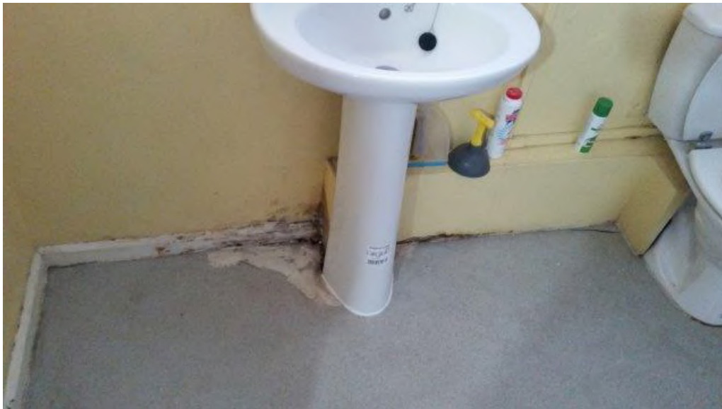
▲ F.43 More bathroom leaks and condensation
