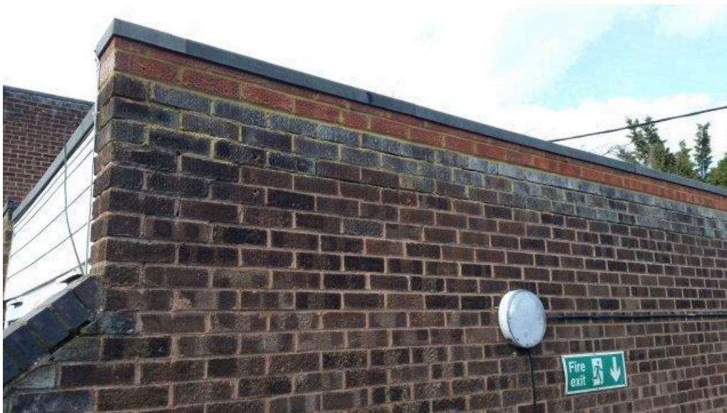
▲ F.12 Some parapets rebuilt due to severity of damage
