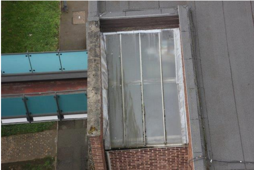
▲ F.09 Poly roof above stairs to be replaced
