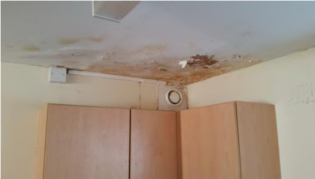
▲ F.41 Void Flat in very poor condition
