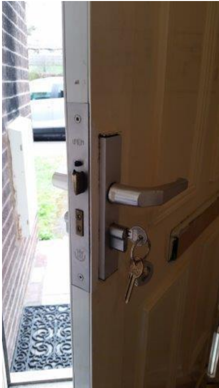
▲ F.35 Problems with doors and locks common
