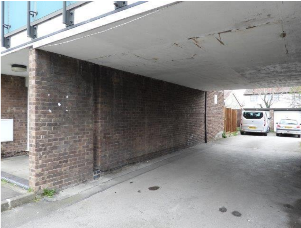
▲ F.45 Fire risk as undercroft ceilings/soffits in poor condition and not fire rated
