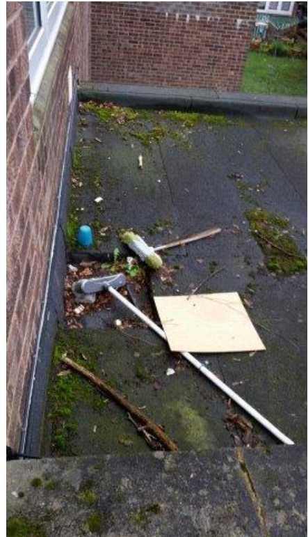
▲ F.06 Low level roofs worse affected
