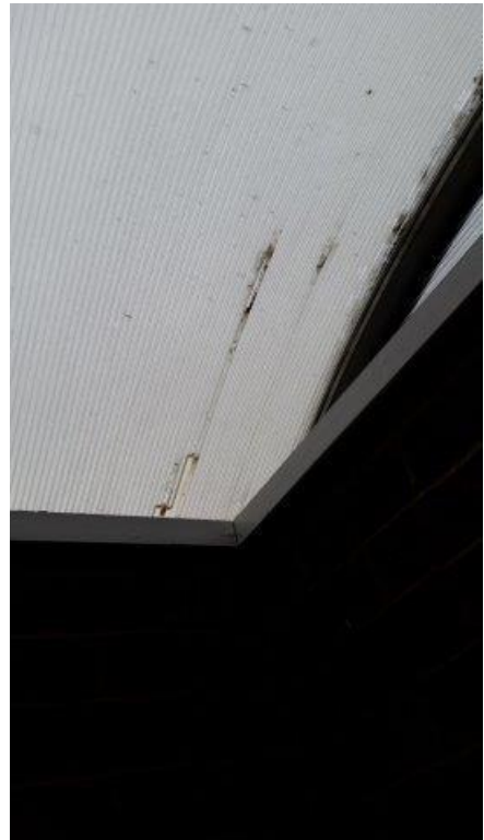
▲ F.08 Rooflight damaged
