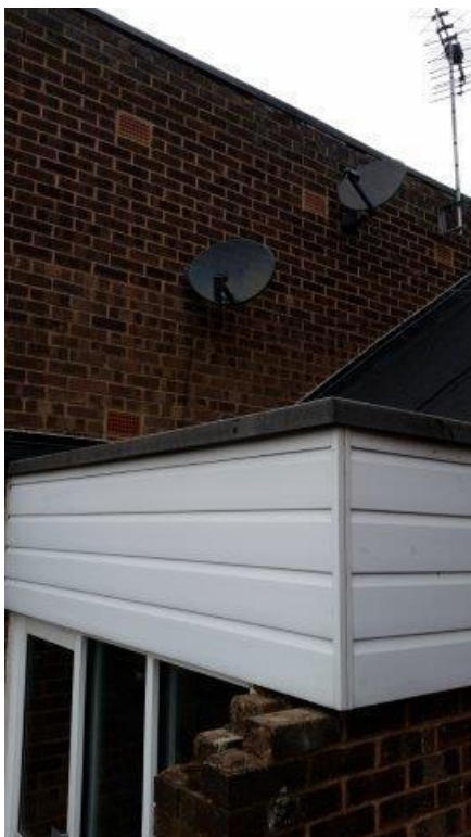
▲ F.20 Air bricks to flat with HRVS
