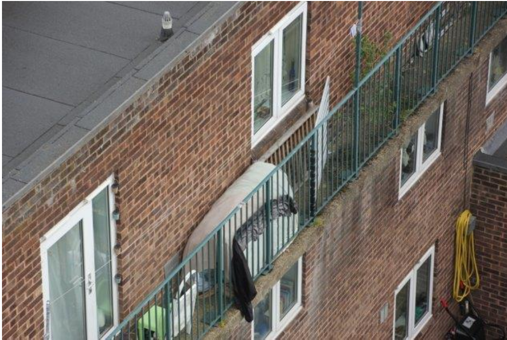
▲ F.11 Balconies saturated and allowing water to penetrate and stain walls
