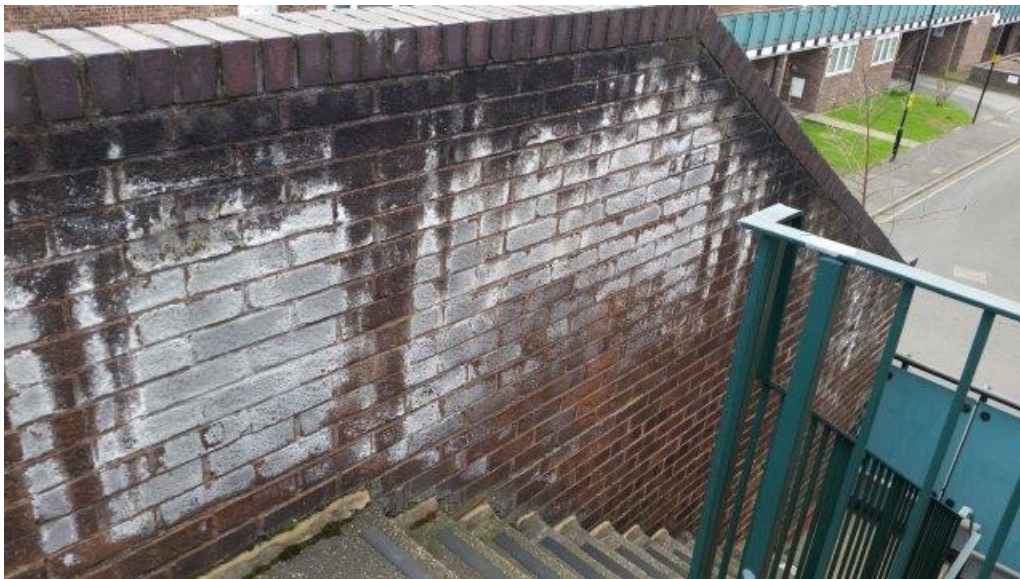
▲ F.14 Exposed areas worse affected. Severe efflorescence shown here.
