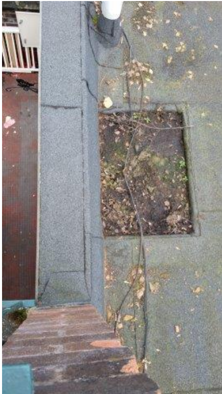
▲ F.05 Blocked gullies
