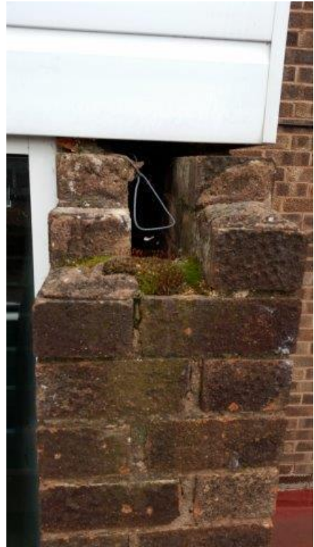
▲ F.16 Coping missing exposing cavity
