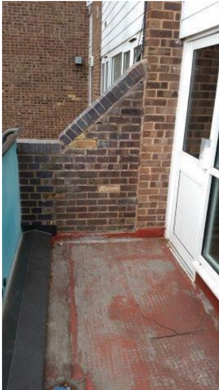
▲ F.15 Parapet dangerously loose
