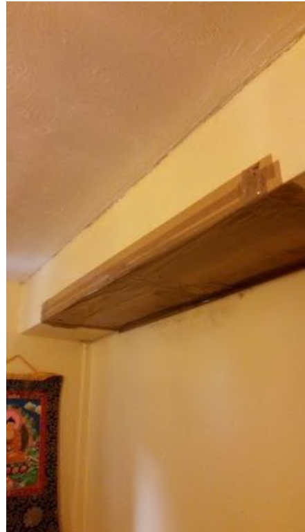
▲ F.36 Water ingress through ventilation ducting
