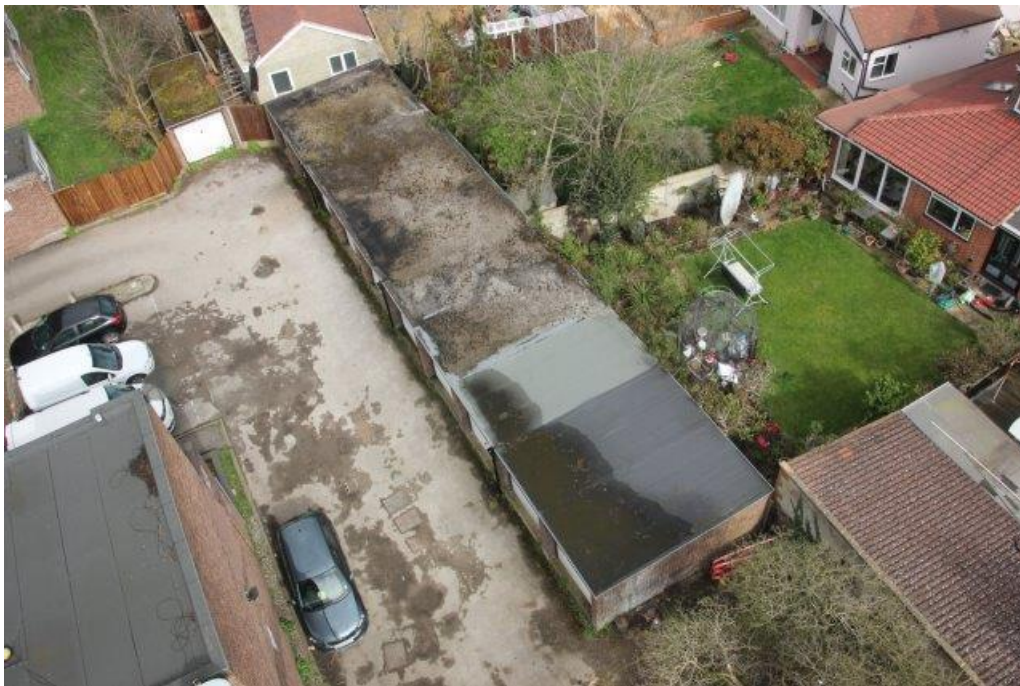
▲ F.28 Garage block roofs saturated, not draining and allowing vegetation to grow
