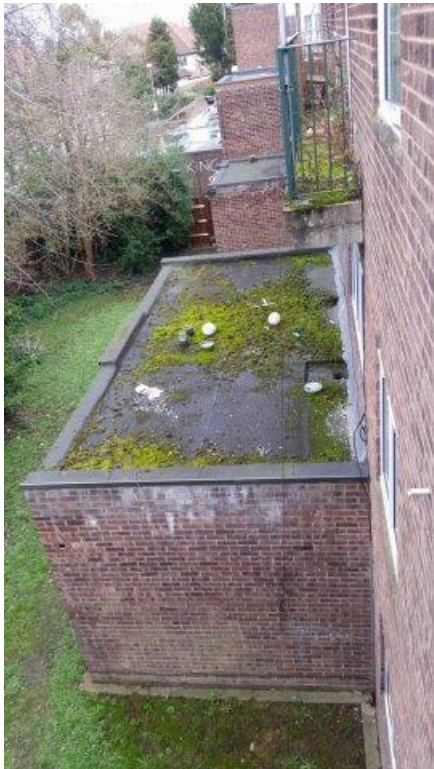
▲ F.07 Vegetation and debris to low roofs
