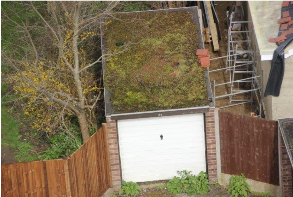
▲ F.29 Garage block roofs saturated, not draining and allowing vegetation to grow
