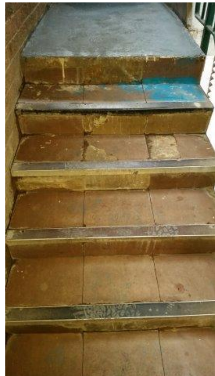
▲ F.26 Flooring tiles in very poor condition
