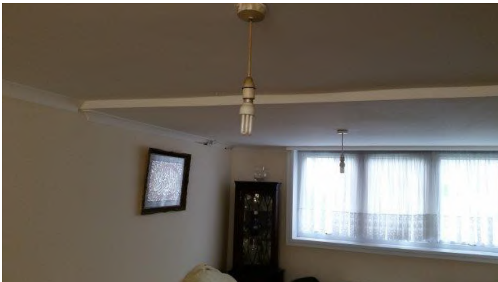
▲ F.40 Bulkhead installed to cover over problems with walkways above
