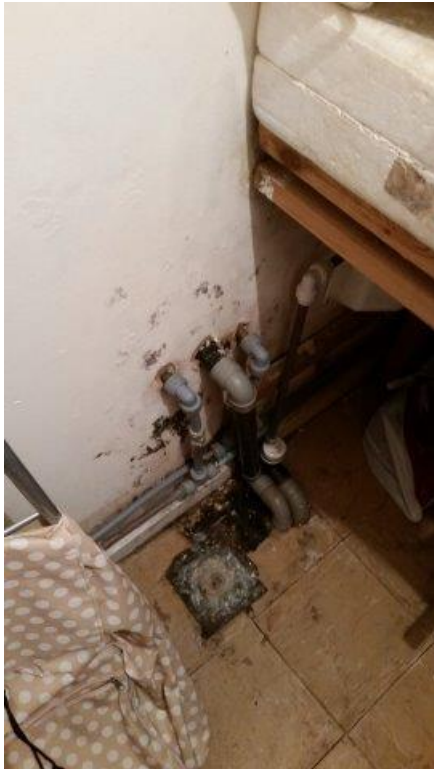
▲ F.38 Leaking pipework
