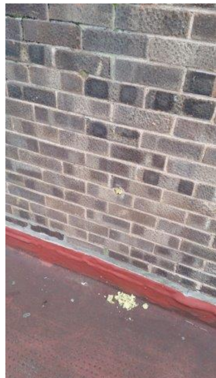
▲ F.21 Cavity wall insulation coming from wall where mortar has "popped"
