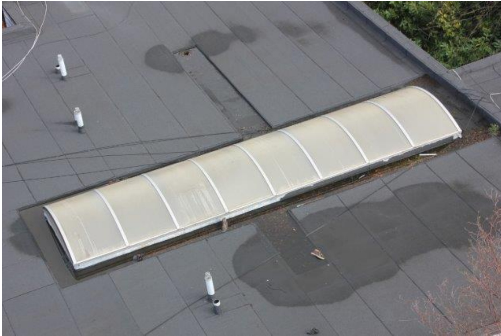
▲ F.03 Gullies and channels completely blocked
