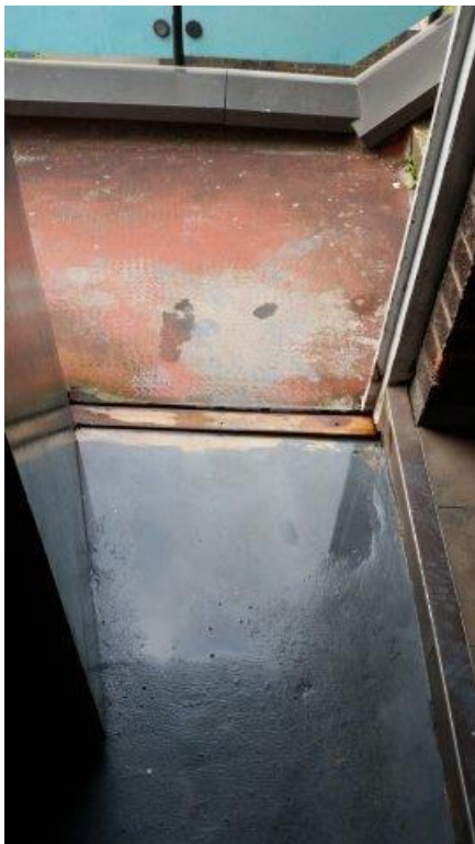
▲ F.25 Inadequate falls and poor detailing allowing rainwater to pond dangerously on landing above stairs.
