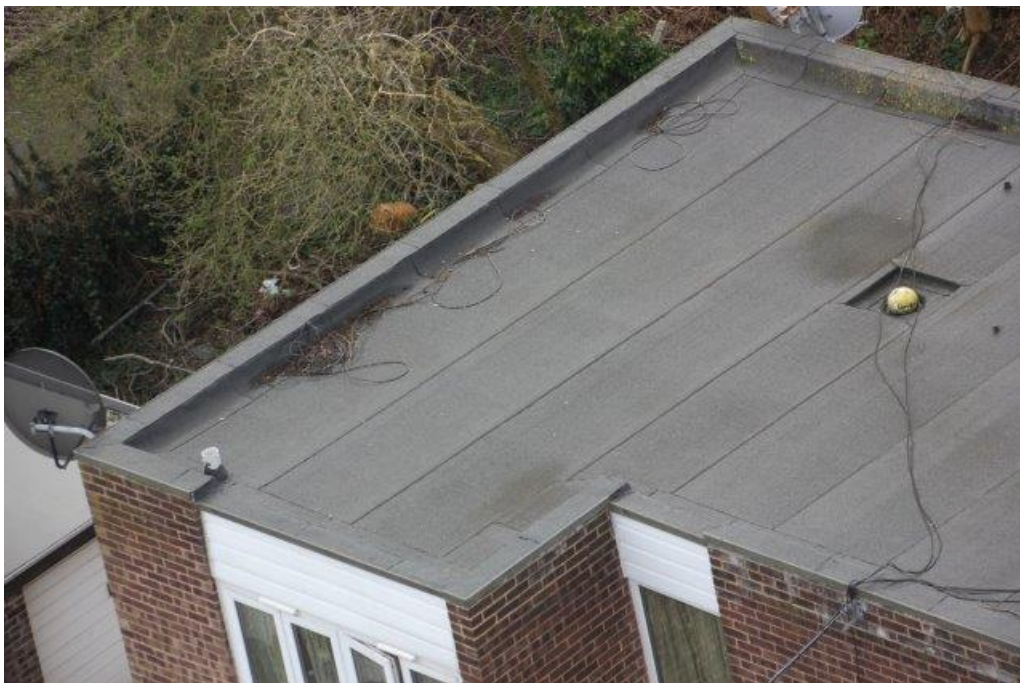
▲ F.04 Blocked gullies and a mess of cabling to all main roofs
