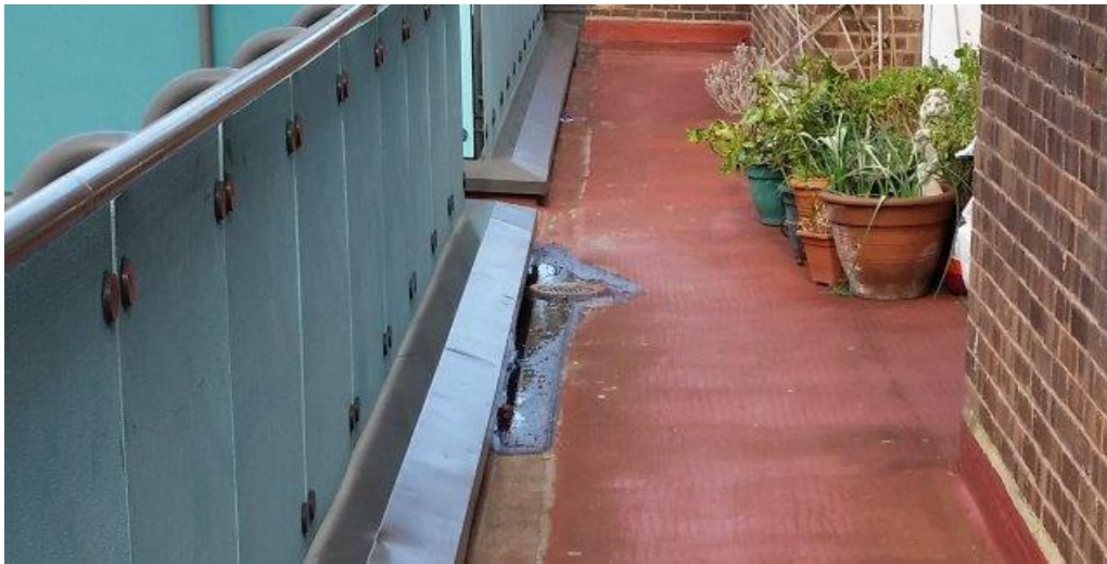
▲ F.22 Poor detailing to walkway gully not allowing water to drain
