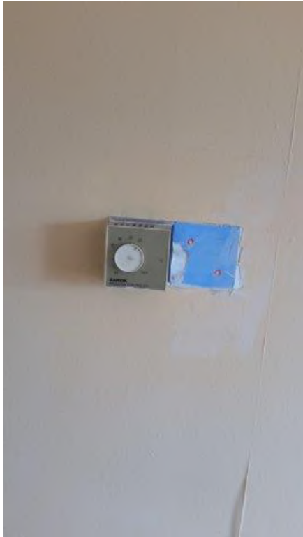
▲ F.33 Redundant fittings left
