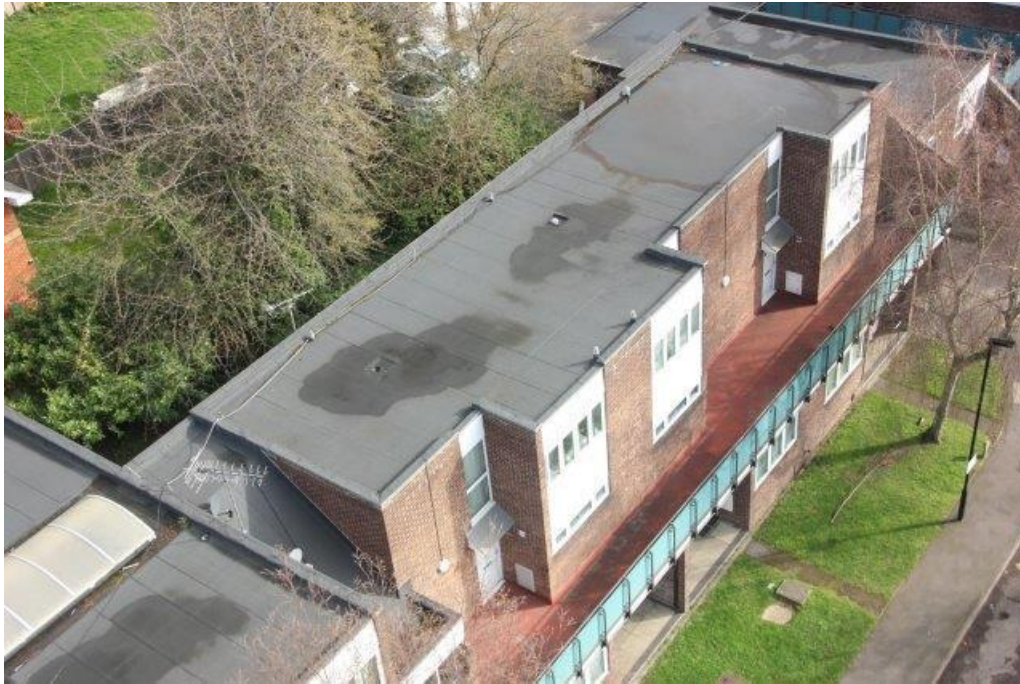
▲ F.01 Severe ponding to main roofs
