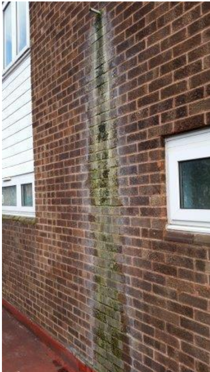
▲ F.17 Condensate pipe staining
