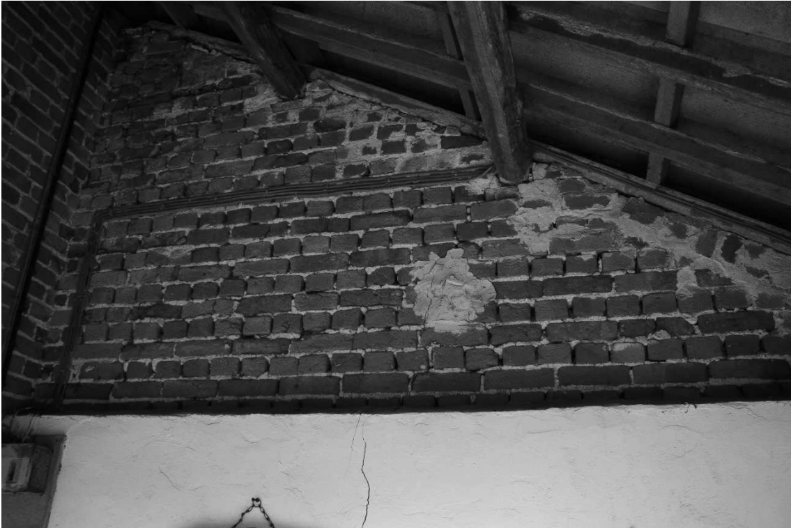
16. Weathering and mortar loss to gable peak of rear offshoot left hand wall
