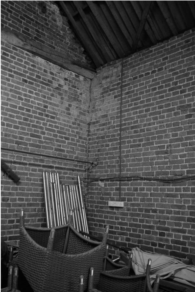
11. Cracking to rear left corner of barn showing remedial tie rod
