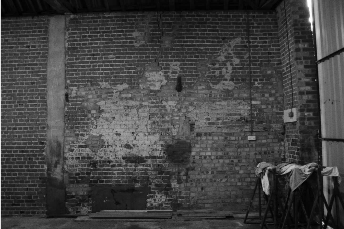
13. Internal cracking to right hand end of rear wall
