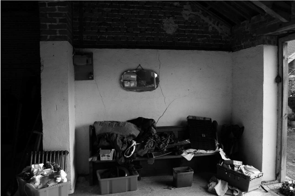
15. Cracking to internal render of rear offshoot left hand wall
