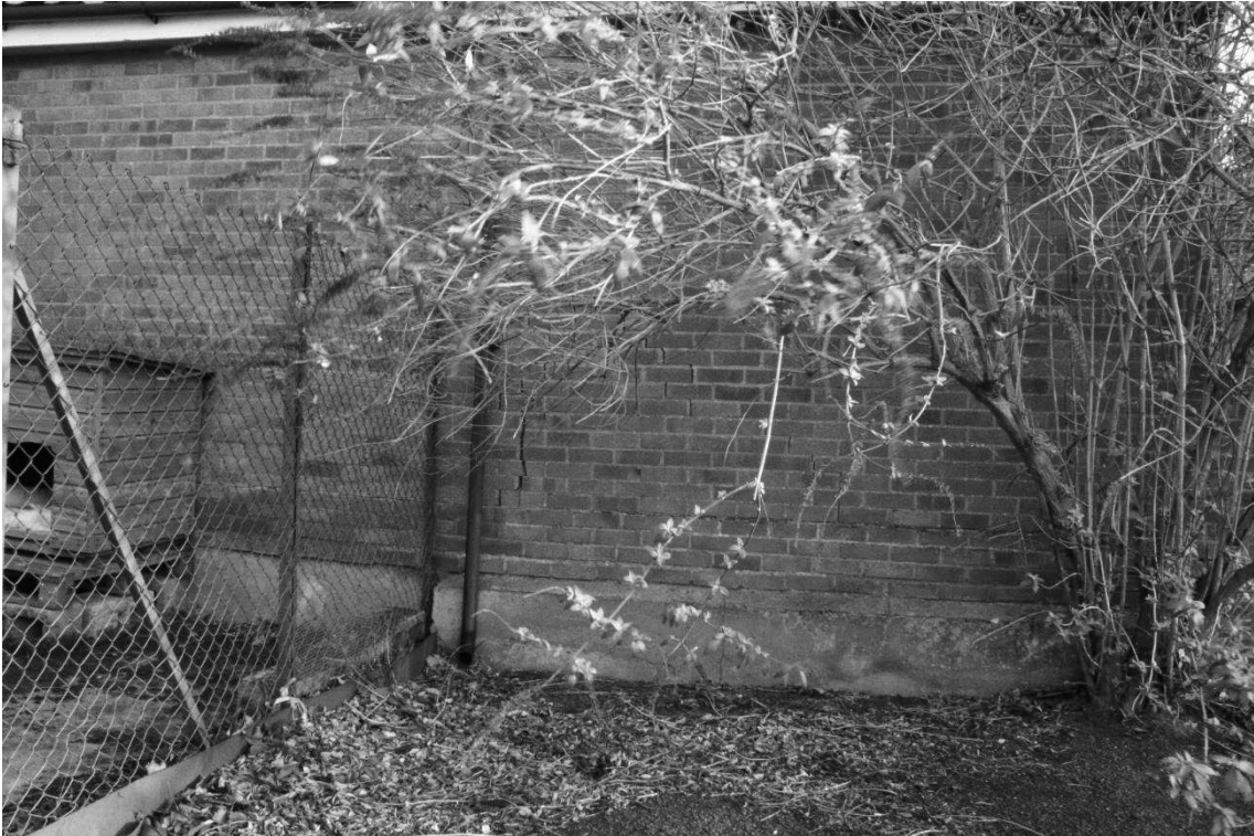
6. External cracking to right side of store
